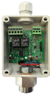
Probe with sensor to be replaced
